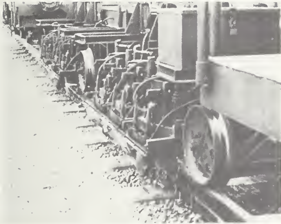
Sparks fly from beneath BART's Speno train as it grinds rail to provide the utmost in rider comfort and safety. Rails were first ground before BART service started, to remove mill scale that could have caused car-control problems.
