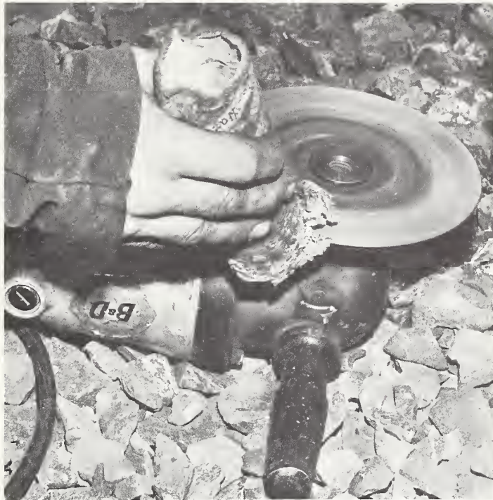
FIGURE 3 APPLYING WAX TO DISC GRINDER TO PREVENT CLOGGING OF DISC BY ALUMINUM
