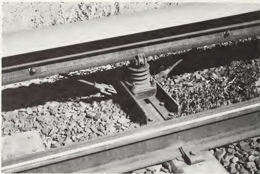
FIGURE 9 CONTACT RAIL ANCHOR ON CONCRETE TIE AFTER FIVE YEARS
