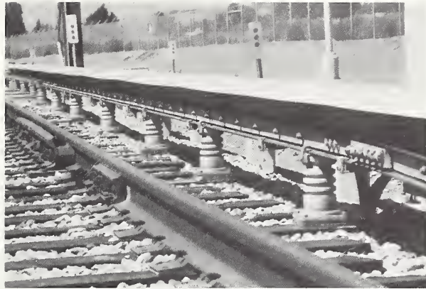
FIGURE 5 CONTACT RAIL WITH BOLTED ALUMINUM SIDE PLATES
