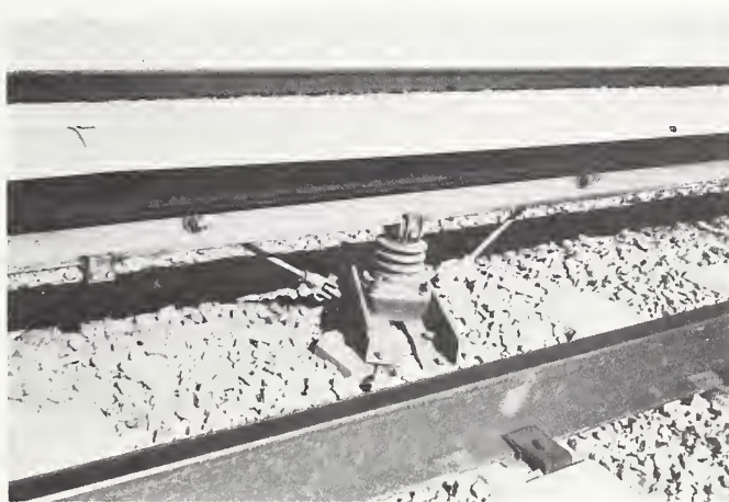
FIGURE 25 BROKEN THIRD RAIL ANCHOR AND CONCRETE TIE
