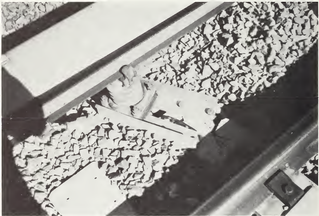
FIGURE 26 CLOSE-UP BROKEN THIRD RAIL ANCHOR AND CONCRETE TIE
