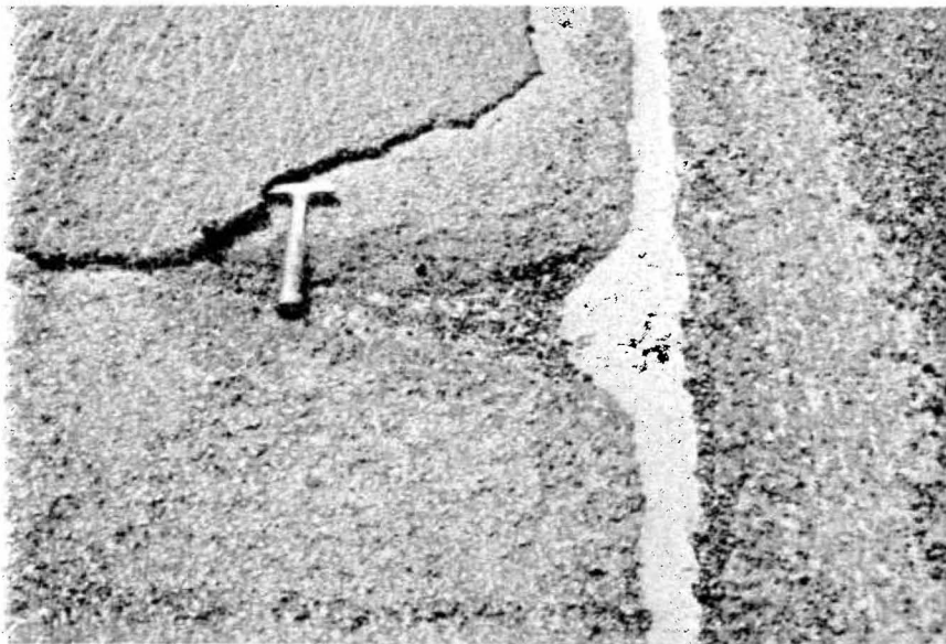
Figure 7 Disbonded slabs of 1967 mix. Surface in foreground is mix placed in 1955.
