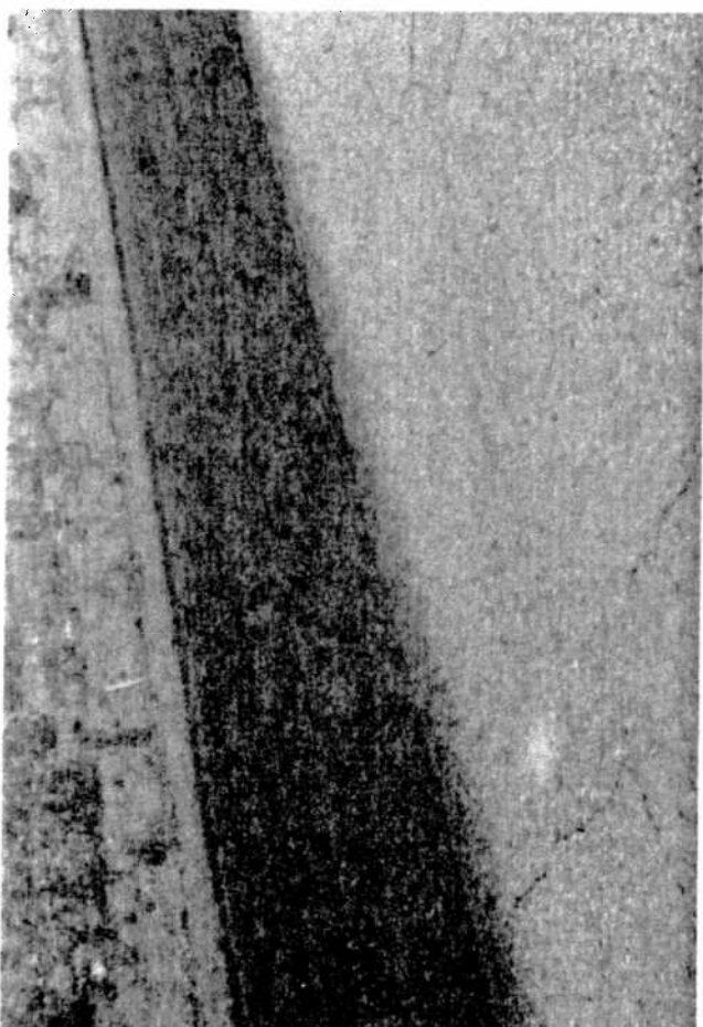
FAR LANE TREATED--NEAR LANE STILL CRACKED
