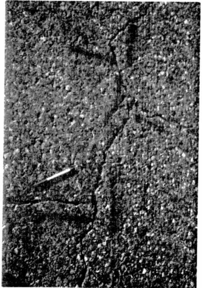
CLOSE UP OF CRACKING & RAVELING
